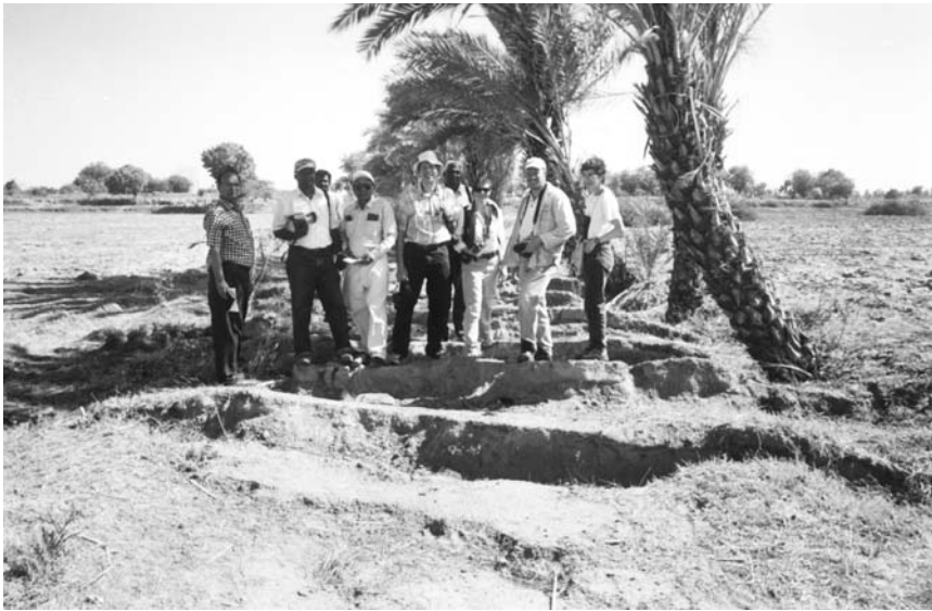
Photograph 5 Step-like lateral spreading on a south sloping road east of the Budharmora uplift.
