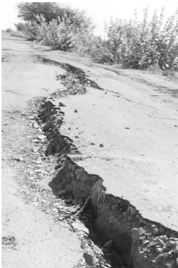
Photograph 8 About 80 cm uplift of the southern side of a road at Chopadwa.
